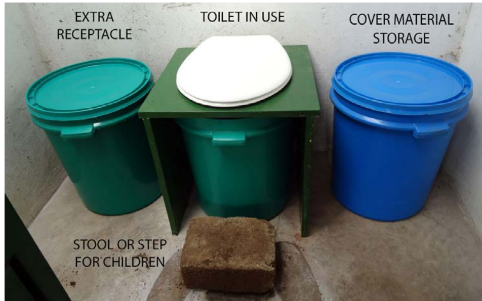
Figure 1-Formerly a pit latrine, a compost toilet system is setup at the Police Barracks School in Moroto, Uganda.
